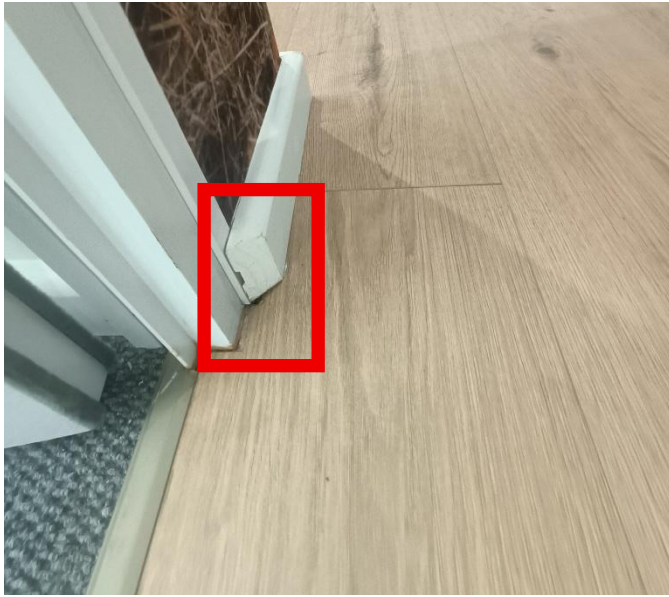
62. Pencils marks on the timber floor to be removed.
