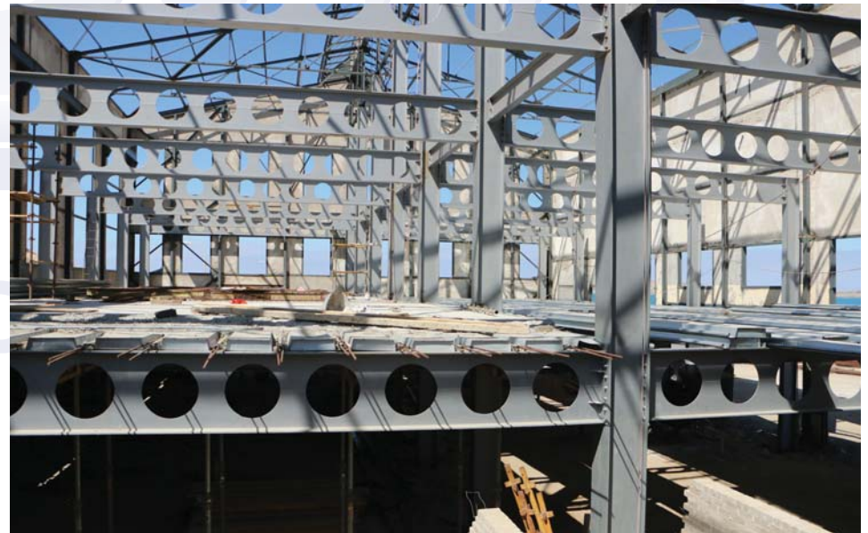
Power Station - Luderitz
