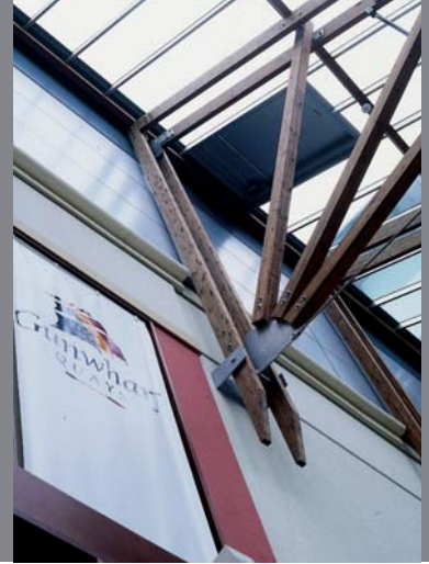
Gunwharf Quays, Portsmouth. Colt OPV controlled Seefires installed into a Colt roof glazing system. Fixed glass smoke curtains are also installed at high level.
