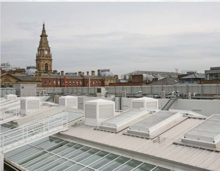
Metquarter Shopping Centre, Liverpool. Colt installed Seefire natural ventilators to provide natural day to day and smoke ventilation on the roof, as well as smoke curtains in the mall.
