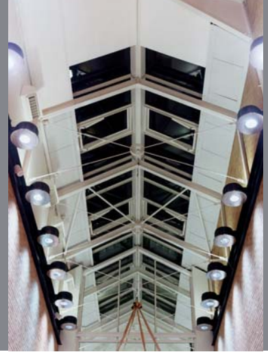
Castle Quay Shopping Centre, Banbury. Kameleon glazed natural ventilators installed into the malls glazing system to provide high level natural smoke and heat extract.
