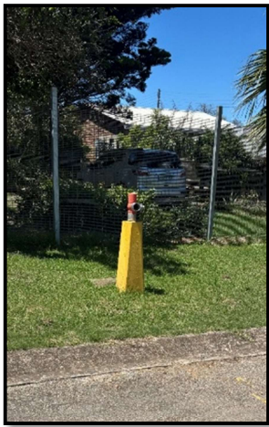
Figure 5: Existing Fire Hydrant
